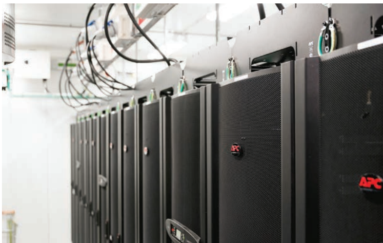
Typowe Data Center (fot. Schneider Electric)
